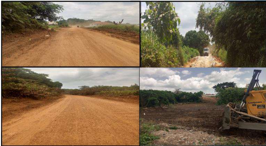
Figure 4: Created access and reshaped feeder roads within the District (GoG, IGF, DACF)
